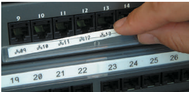
Punch Block & Patch Panel Labels
