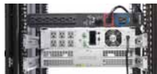
HotSwap MBPs rackmounted horizontally in rack
