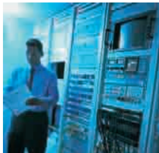
Servers, data storage and network equipment
